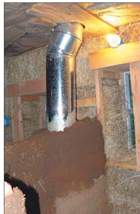
The rocket stove's ductwork helps spread heat around and vents exhaust to the outside. Photo by Paul Hanson.
